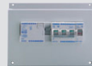
FI-safety switch (4-pol. 40A/0.03A) Fuse (3-pole 35A), fuse (1-pole 16A)
