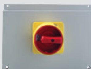
Emergency stop main switch
