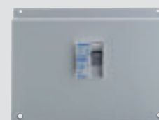
FI safety switch (2-pol. 25A/0.03A)
